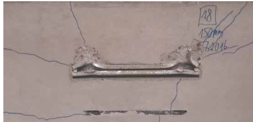
Fig. 10 Typical failure mode for both standard and rebar channels in the experimental investigations.
