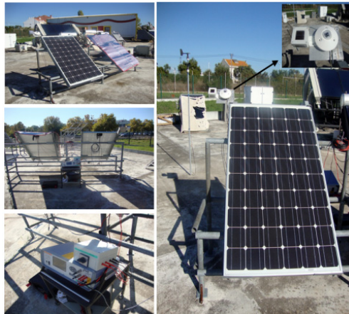
Fig. 3. Photovoltaic facility at the LNEG.
