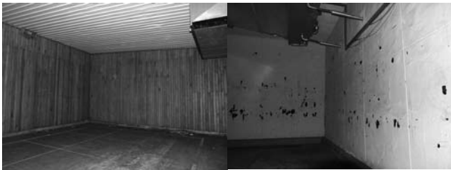
Fig. 2. Detail of two of the small cold chambers before demolition (the first with ICB protected by wood; the second with painted ICB).
